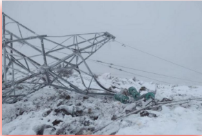
July 2020, Chubut, Argentina. 55 high-voltage transmission towers were knocked down.
